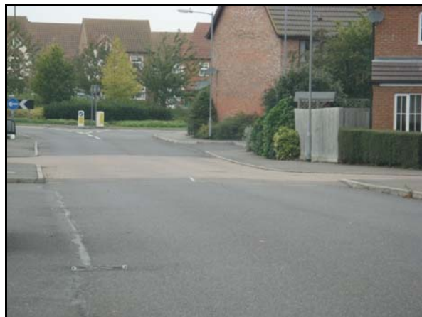
Speed Table on Woodcock Road and Nightingale Close with lack of road markings
